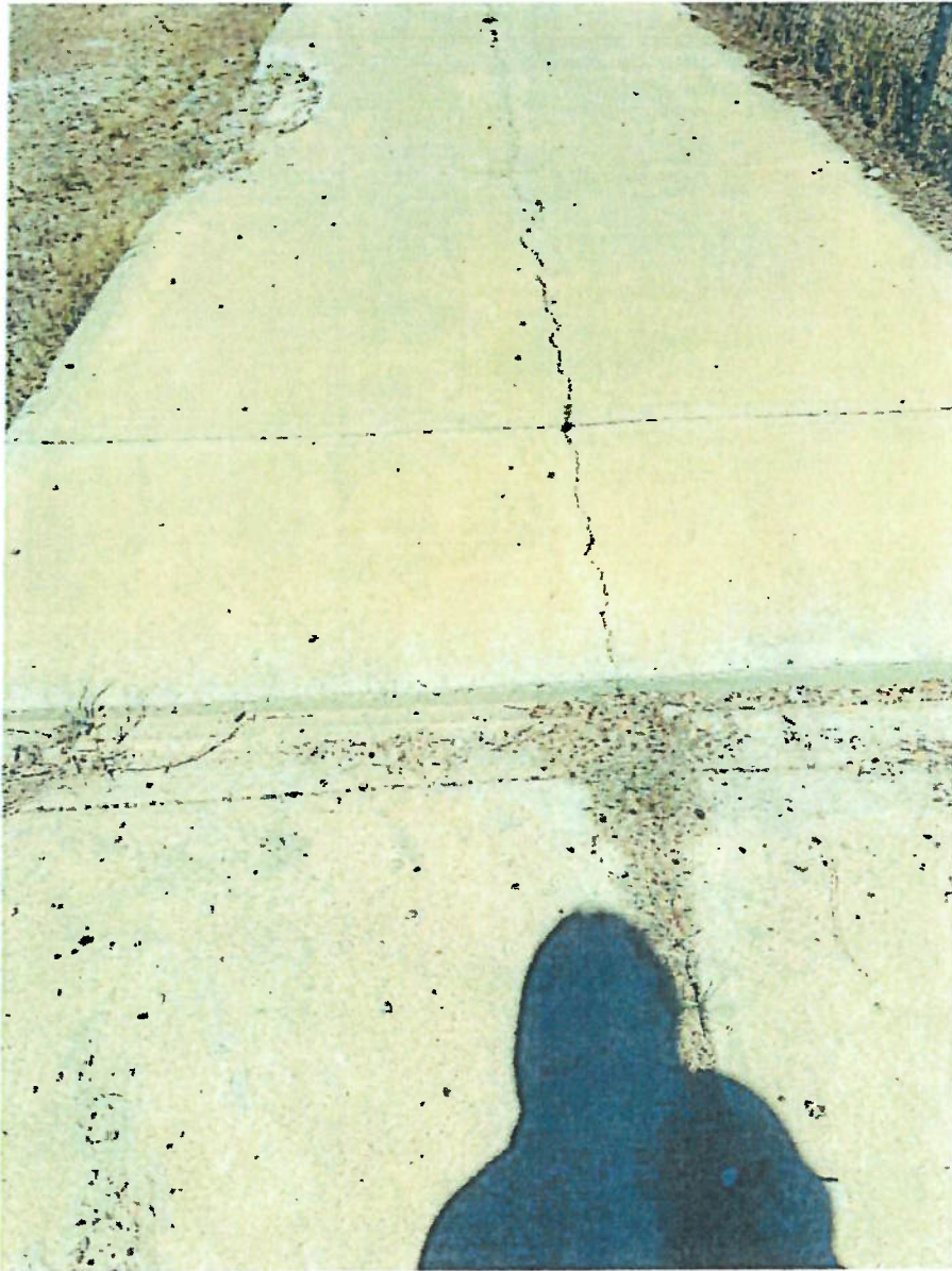
Photo 3: Step up in the middle of the sidewalk
