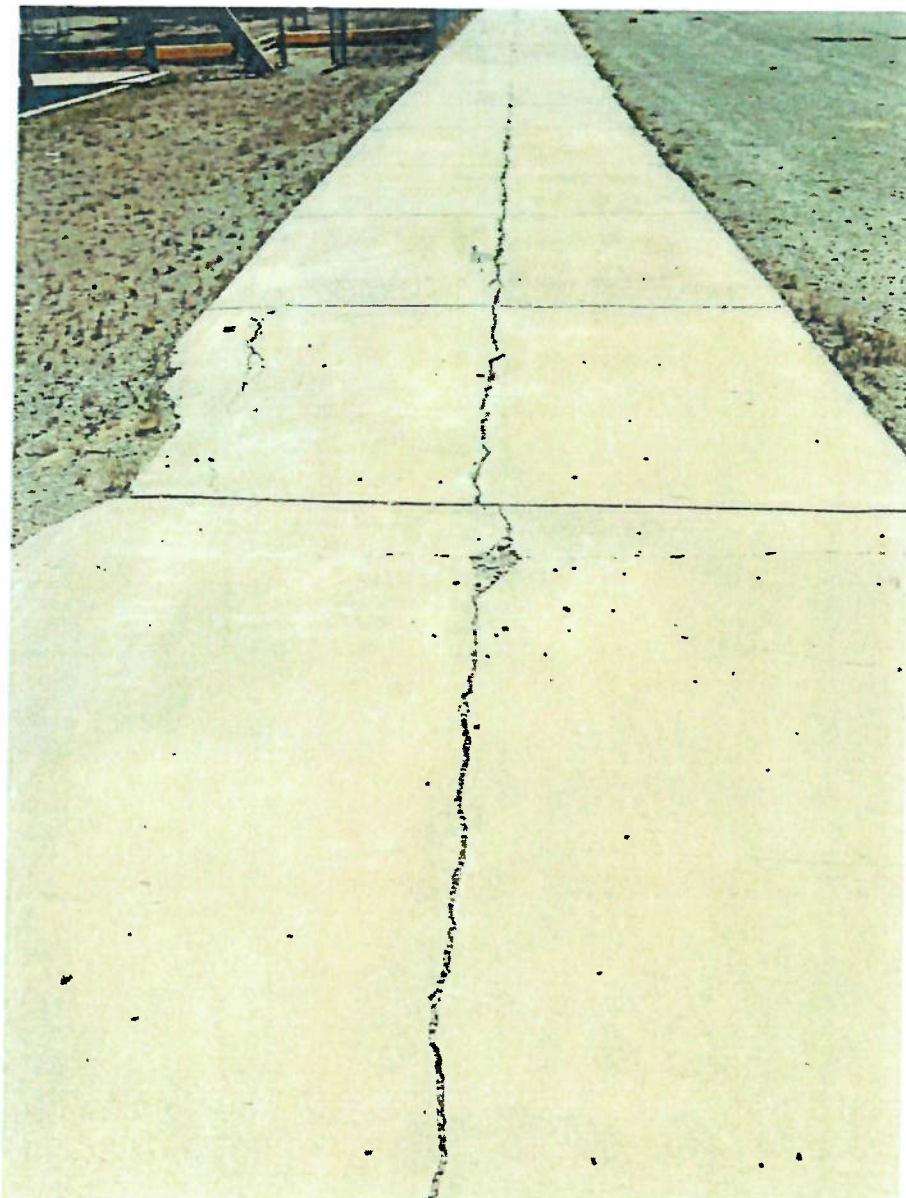
Photo 4: Large crack running down the length of the sidewalk
